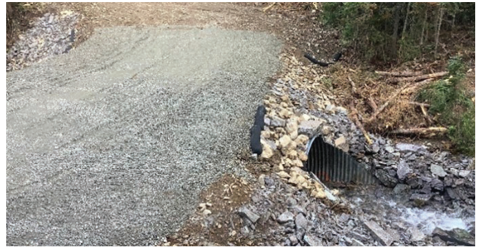
Stream crossing installed to minimize sediment delivery to the stream and provide fish passage.
