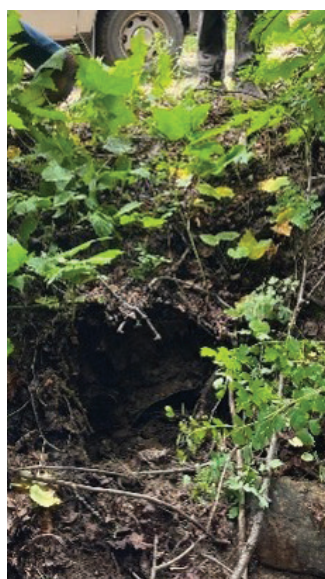
Culvert that needs cleaning
