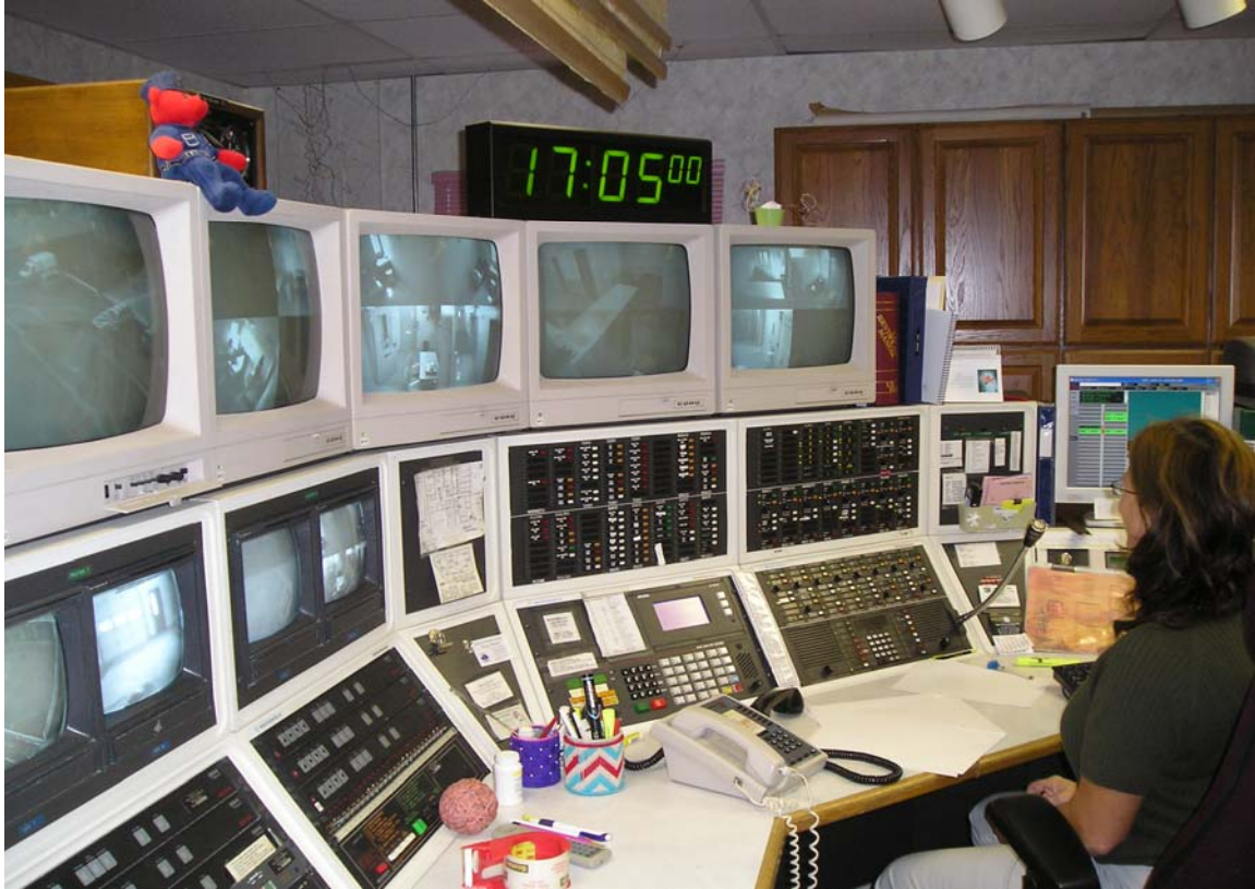
Dispatch Center in Baker
