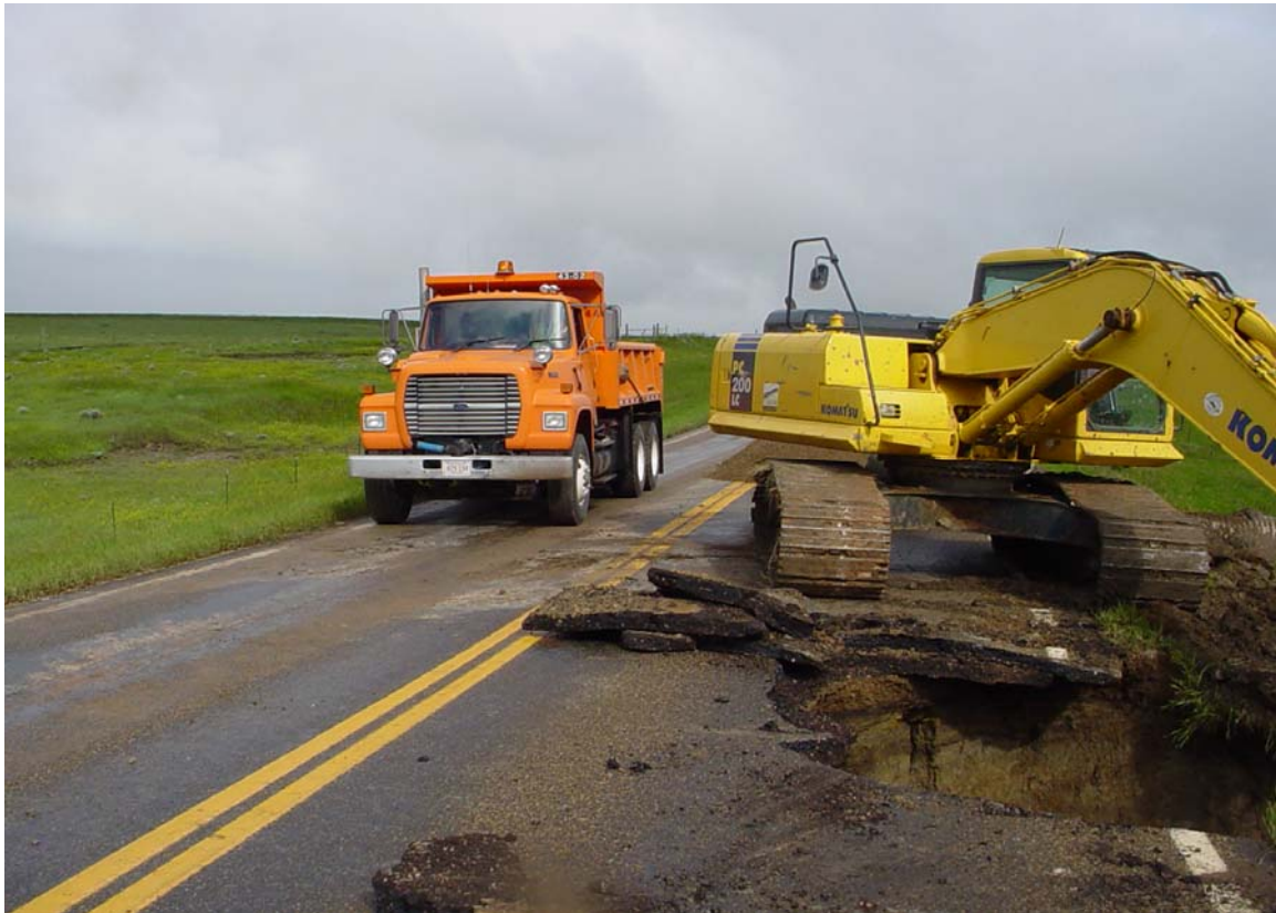
Flood Damage on Route 322 SE of Baker, June 28, 2005
