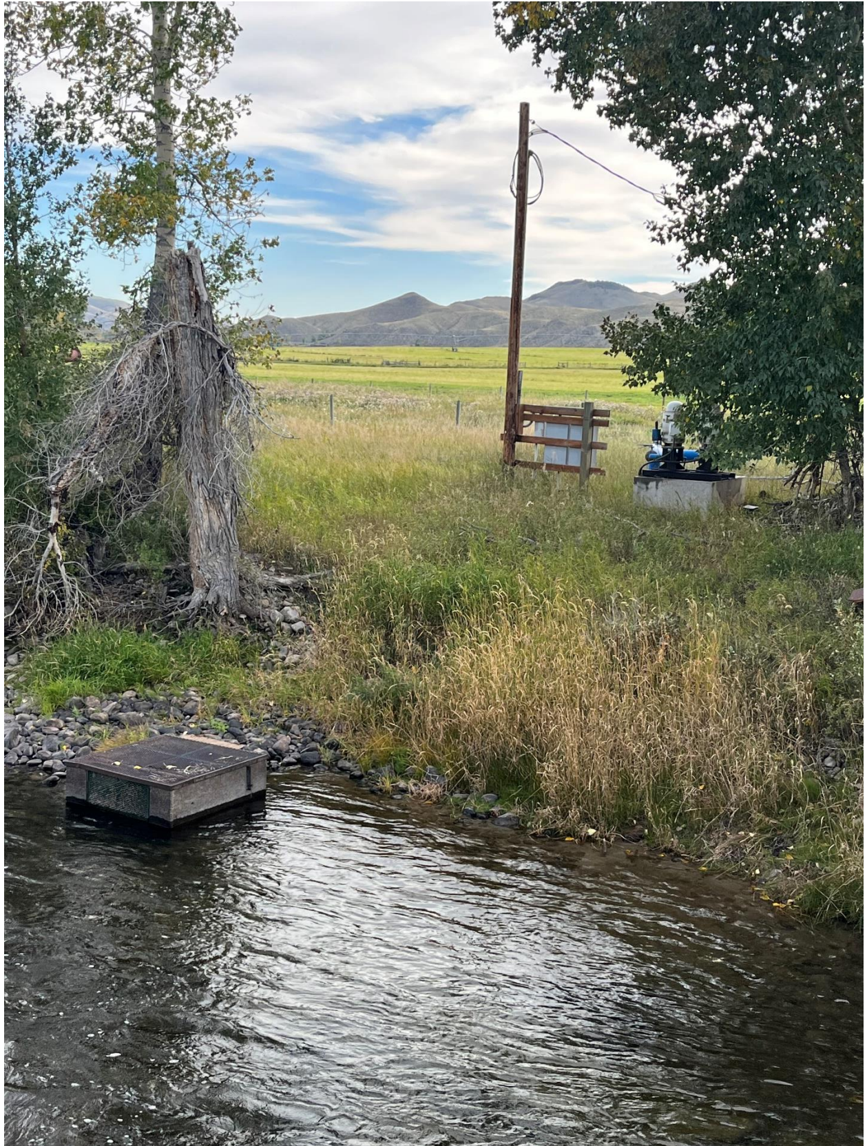
Example of similar pump site installed on Big Hole River.
