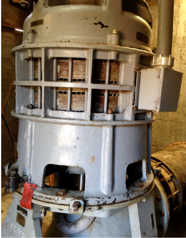
Photograph 34: Crow Pumping Plant pump motor.
