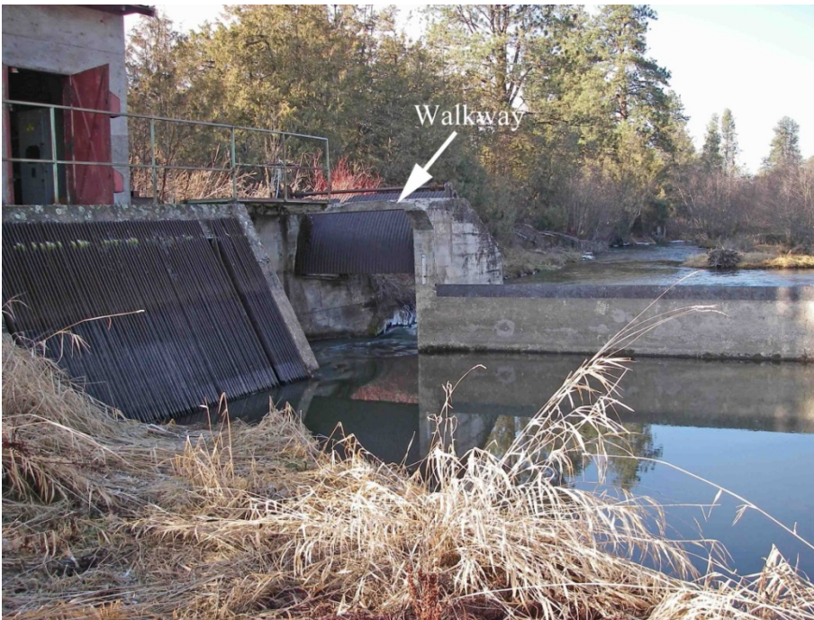
Photograph 33: Looking downstream at the Crow Pumping Plant diversion dam with steel radial gate at the left end. The arrow points to the concrete walkway, which should have a handrail installed along the upstream and downstream sides.
