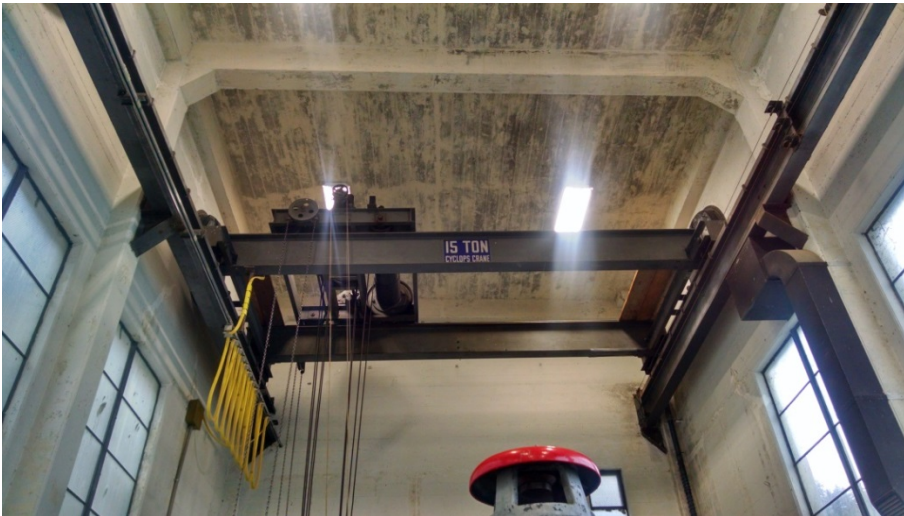
Photograph 30: Flathead Lake Pumping Plant crane.
