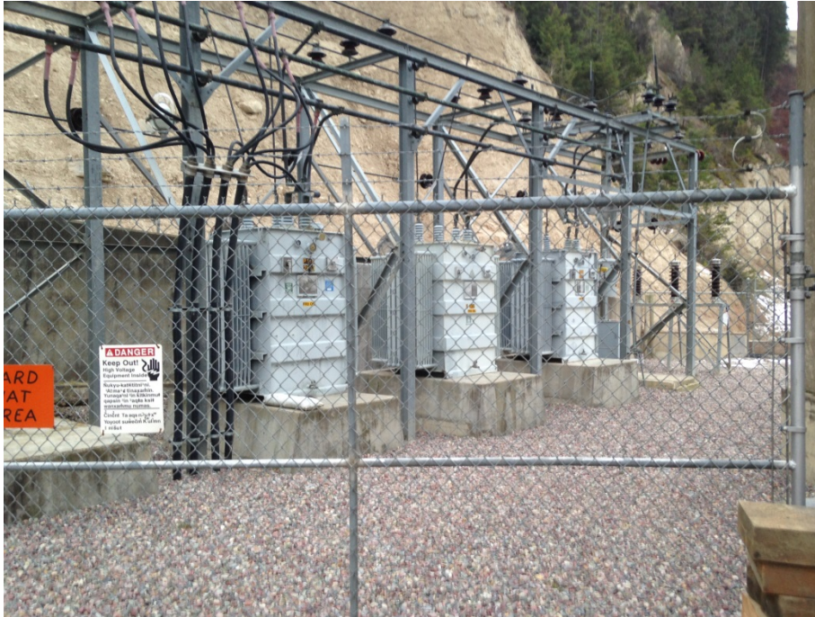
Photograph 11: View of Flathead Lake Pumping Plant substation main transformers.
