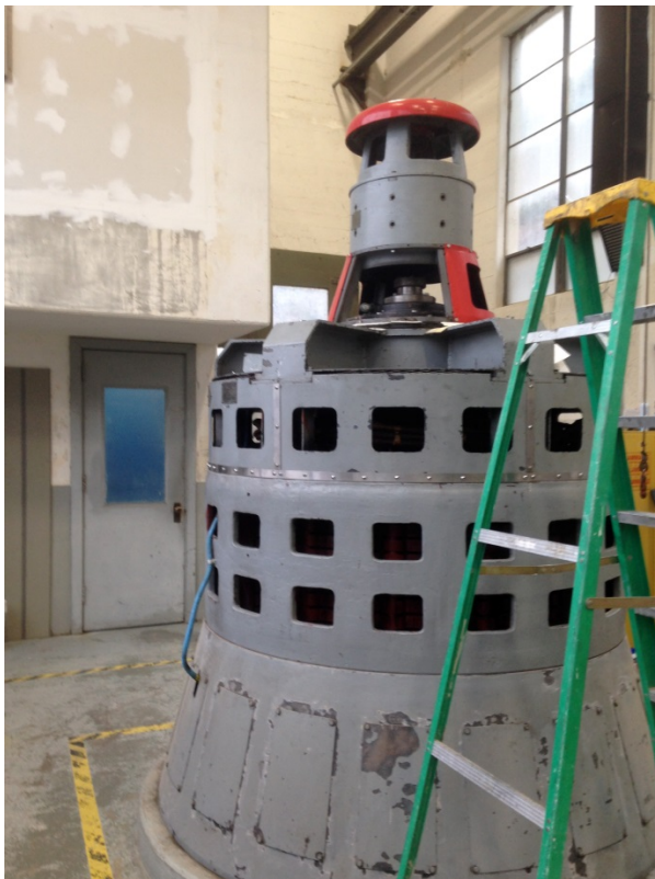
Photograph 16: 3,000 horsepower pump motor.
