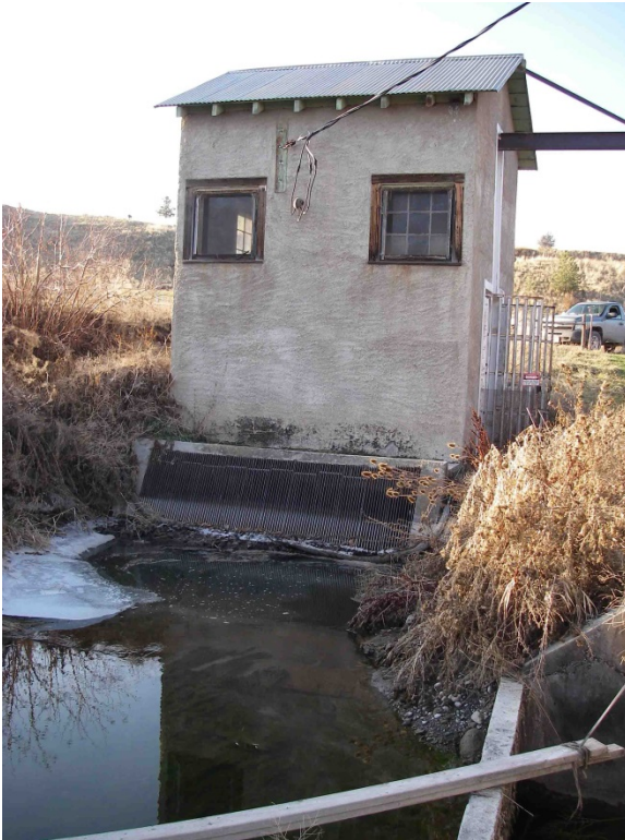
Photograph 35: Reavis Pumping Plant building and intake structure.
