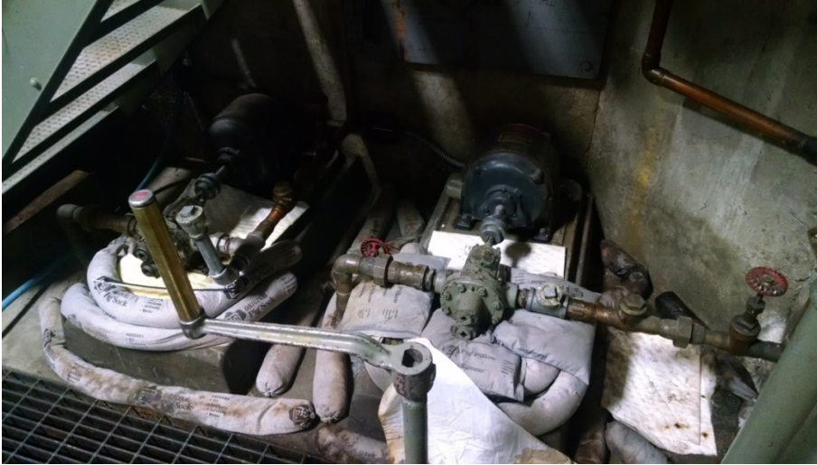
Photograph 29: Bearing Oil Pumps.
