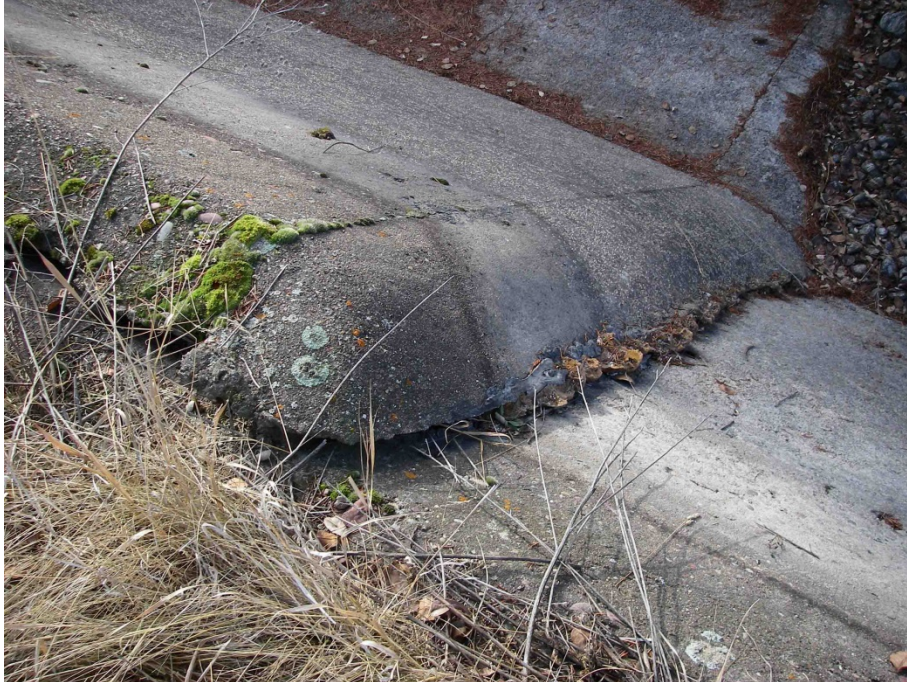
Photograph 9: Looking at the gap between the second and original concrete liners.
