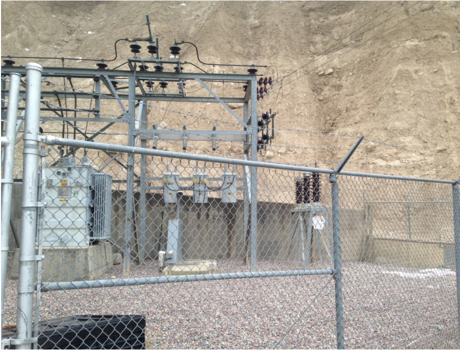
Photograph 10: View of Flathead Lake Pumping Plant substation auxiliary transformer and disconnects.
