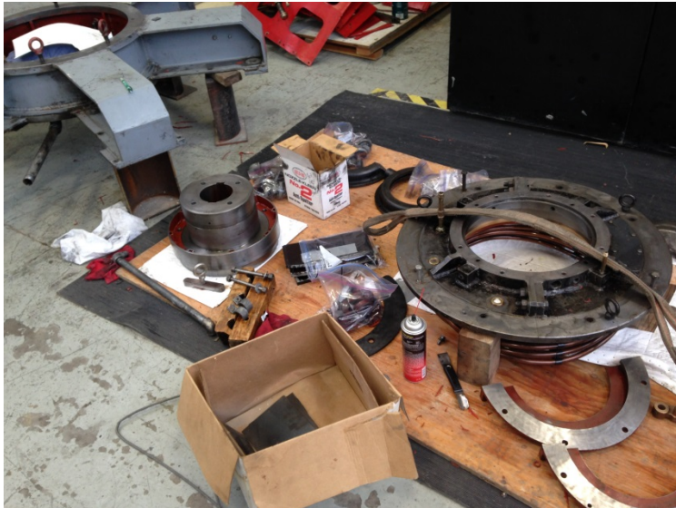
Photograph 15: Flathead Lake Pumping Plant brush assembly and upper bearing parts.
