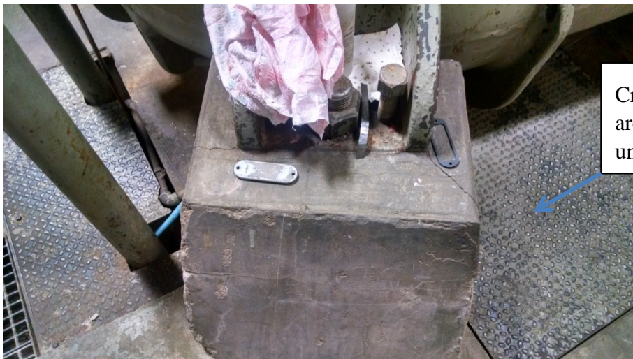
Photograph 28: Cracks on Unit 3 pump mounts.
