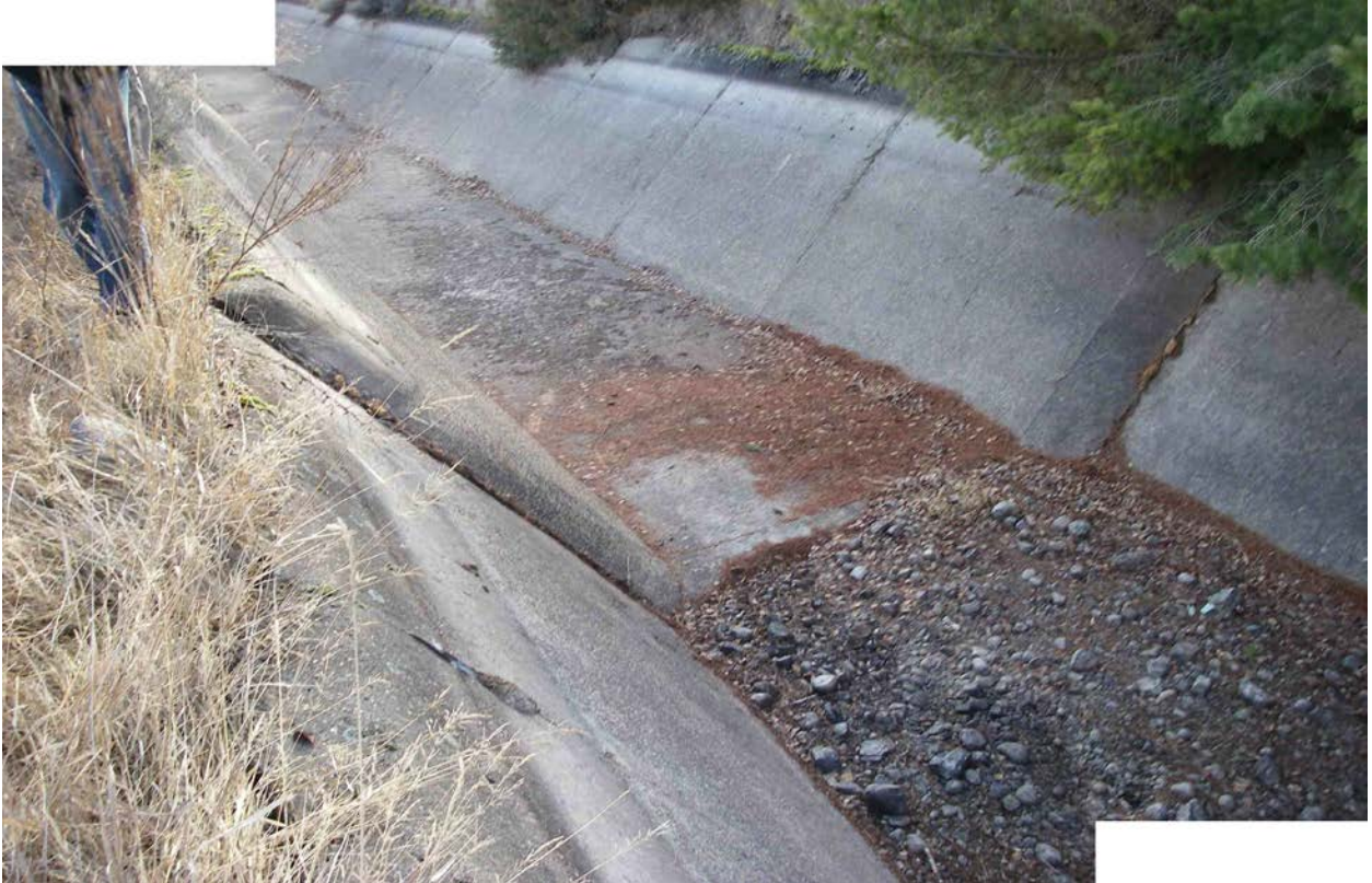
Photograph 8: Looking at the portion of the canal from the Flathead Lake Pumping Plant with a second concrete liner.
