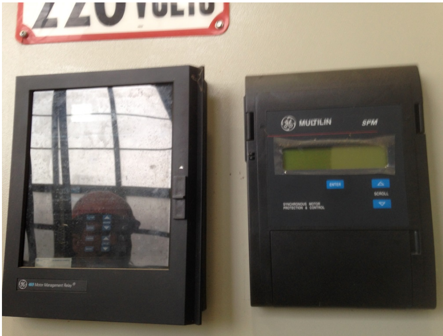
Photograph 25: Flathead Lake Pumping Plant synchronous motor excitation system (Multilin).
