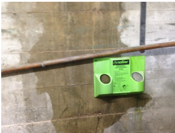
Photograph 24: Looking at missing PPE near the station service batteries.
