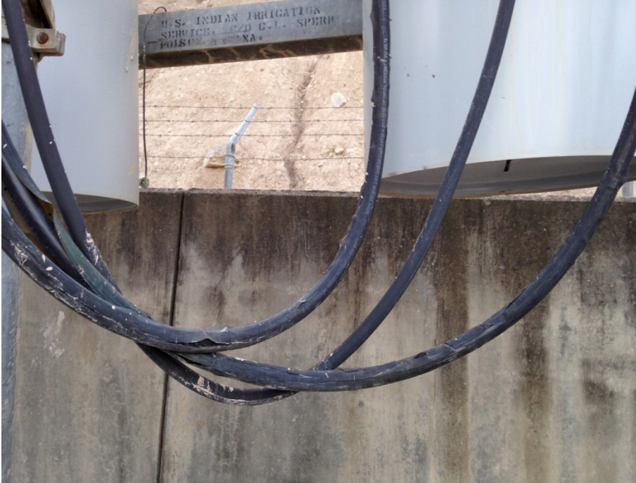
Photograph 13: Photo shows deterioration of cables in substation.
