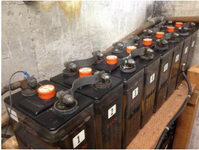
Photograph 23: Flathead Lake Pumping Plant station service battery system.
