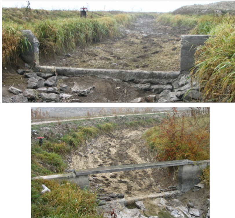
Figure 15. Examples of existing check structures along the MA Canal. Photos from HKM 2008 report (top photo CH-243, bottom photo CH-245)
