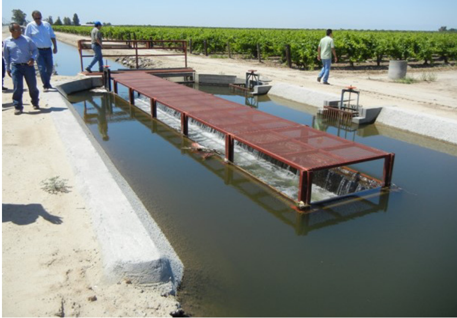
Figure 19. Somewhat similar LCW in Fresno ID, but lacking the side sluice gates and the tapered configuration of the LCW itself (although the banks are tapered). This illustrates a construction technique for tying the walls together for strength, and providing access for operators to clean off the weir crest.
