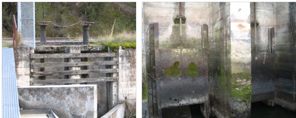
Figure 11. MA Canal headgates. Photo from HKM 2008 report (DD-12).
