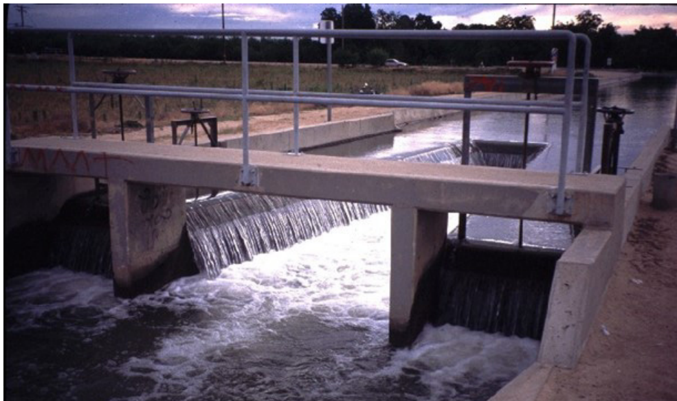
Figure 18. Somewhat similar LCW installed at Turlock ID
