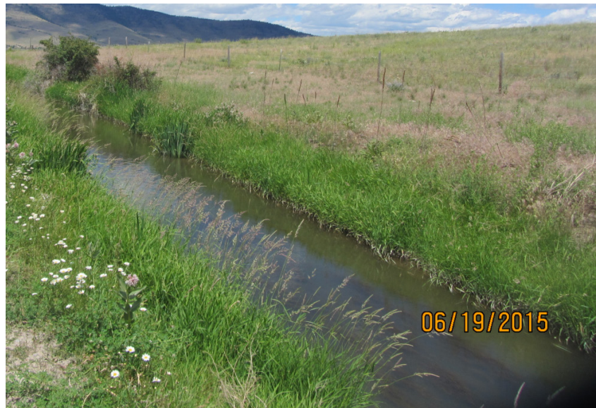
Figure 14. Example of existing condition of the MA Canal. Picture shows a large amount of aquatic growth in the canal.
