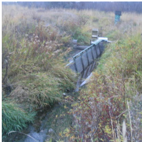
Figure 6. Fish screen installed downstream of the Mission H Canal headgate. Photo from HKM 2008 report (HG-55).
