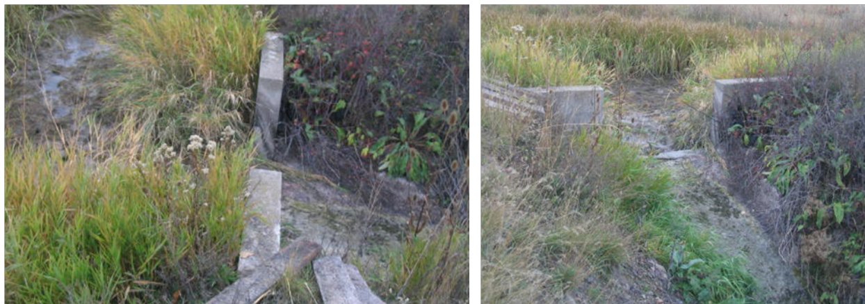
Figure 8. Existing check waste in the Mission H Canal approximately 1.3 miles downstream from the canal diversion. Photos from HKM 2008 report (CW-29).
