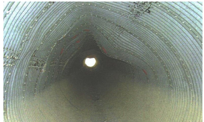
Figure 6. Deformation in a CMP Conduit [1].
