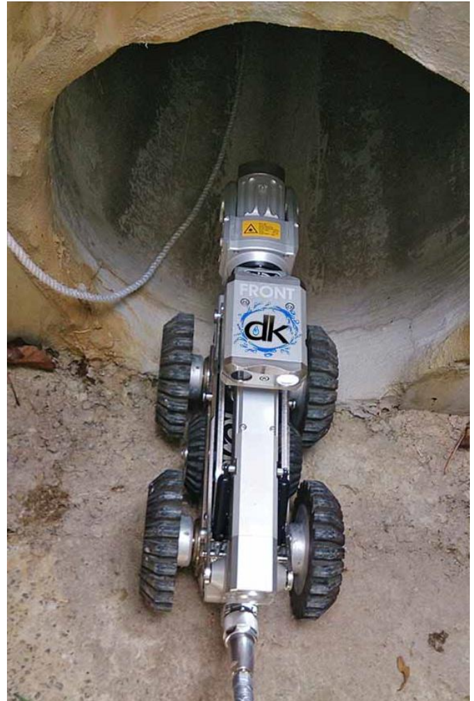
Figure 2. CCTV Camera on a Pipe-Crawler Being Inserted into a Conduit (courtesy Drains Kleen).
