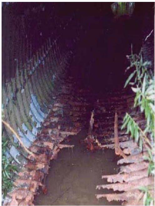
Figure 9. Major Corrosion in a CMP Conduit [2].
