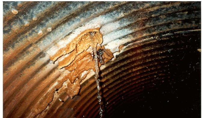
Figure 8. Moderate Corrosion in a CMP Conduit [1].
