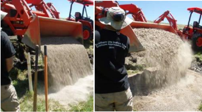
Figures 2a and 2b. Conventional Filter Construction: Placing Sand Filter (Left) and Ballasting With Gravel (Right) at Bureau of Reclamation Dam [2].
