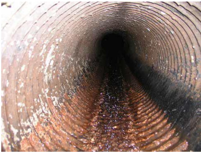
Figure 7: Minor Corrosion in a CMP Conduit [5].
