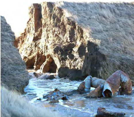
Chouteau County dam that failed in 2011
