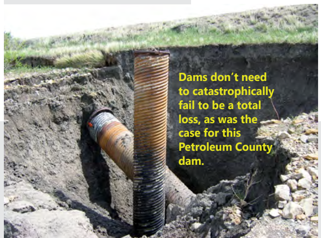
Petroleum County dam in distress
