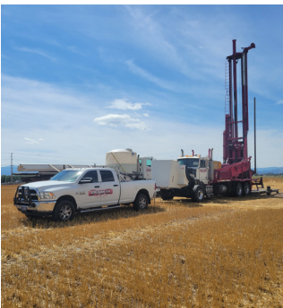
Coldwater Drilling and Pumps, Arlee MT
