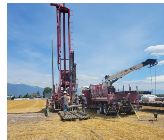
Coldwater Drilling and Pumps, Arlee MT
